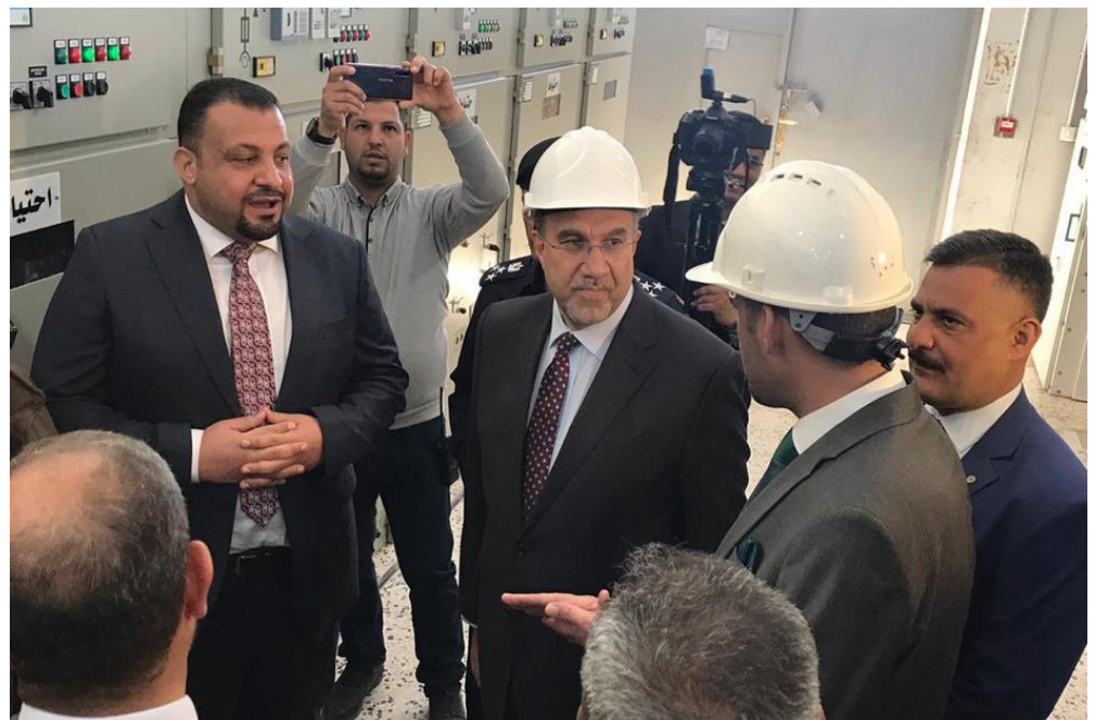
Electricity Minister Luay al-Khatteeb visits a power plant in Fallujah. (Ministry of Electricity)
