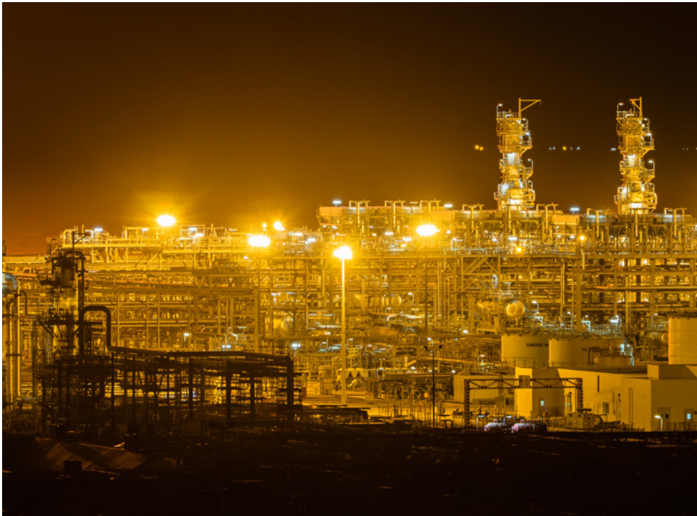
A night view of the Badra oil field, operated by Gazprom Neft. (Gazprom Neft)
